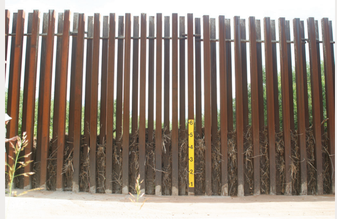
Debris clogging the space between border wall bollards in the San Pedro Riparian National Conservation Area. 2012. Scott Nicol.
