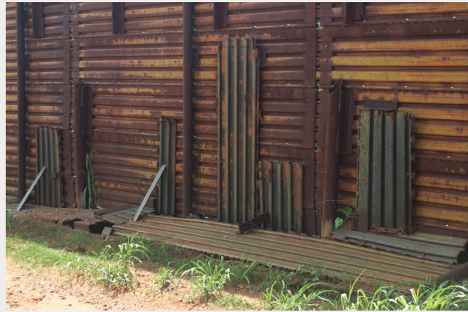
Multiple patches on border wall near Naco, Arizona. 2012. Scott Nicol.
