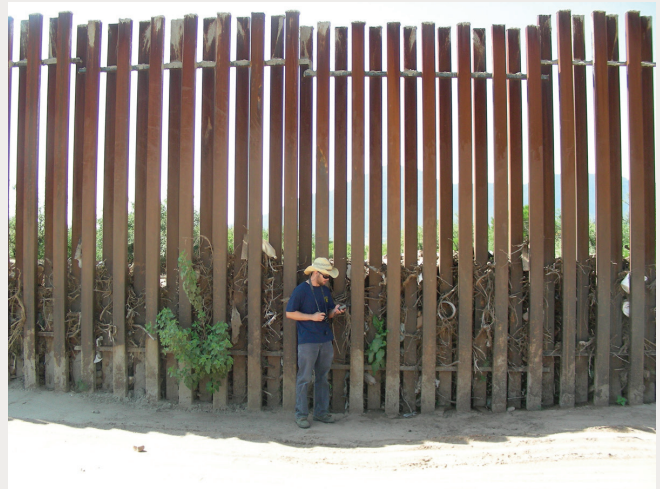
Debris backed up behind a bollard border wall in Arizona. 2007. Bureau of Land Management.
