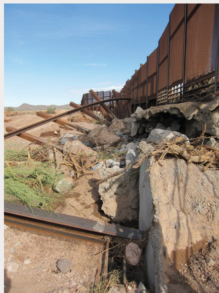
Border wall washout in Organ Pipe Cactus National Monument. 2011. National Park Service.
