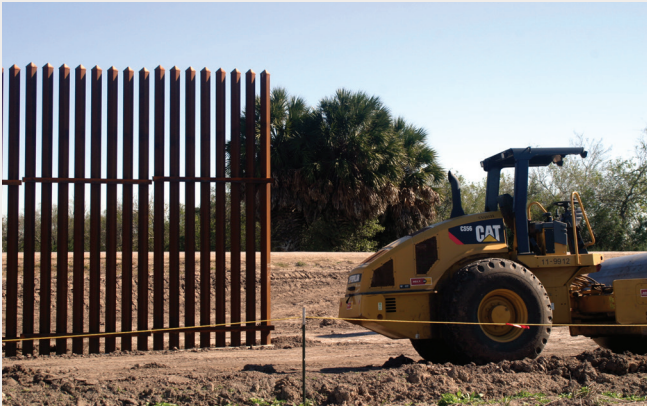
Bollard border wall north of Sabal Palms Audubon Sanctuary under construction. 2010. Scott Nicol.
